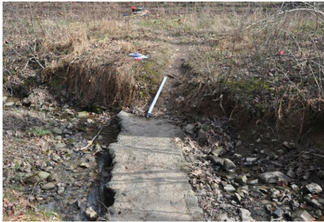
Photograph 8: Eroding sewer crossing before construction
