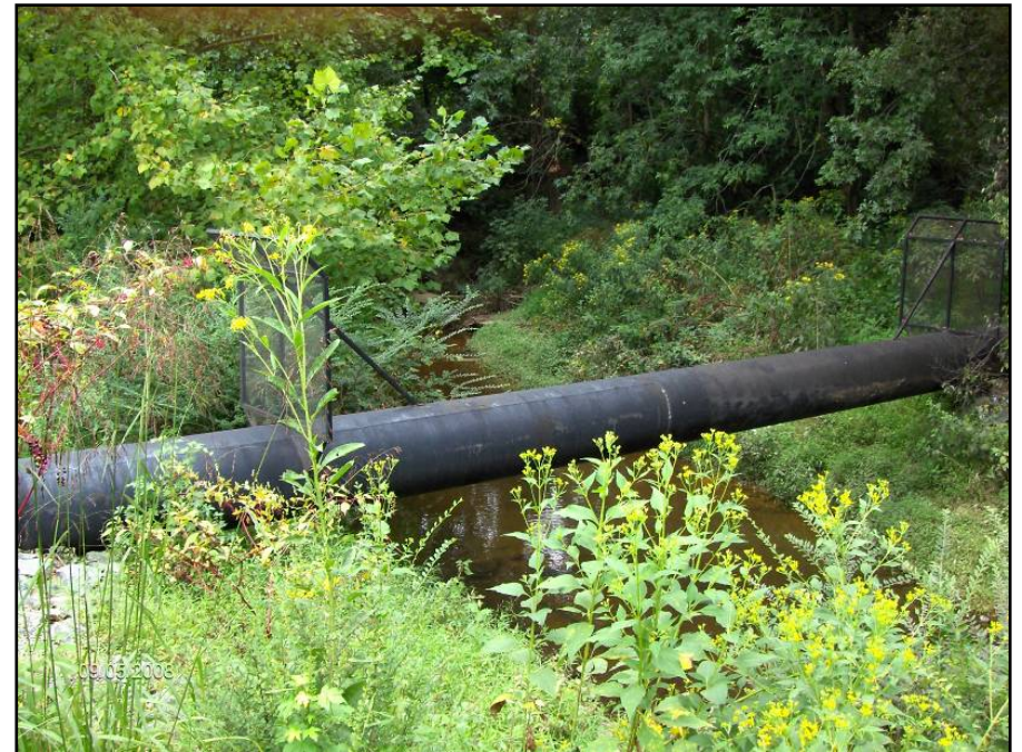
Existing OWASA sanitary line crossing Morgan Creek at the south end of the Canterbury Townhouse community. OWASA has added fencing to each side of the line to discourage pedestrian crossing.
