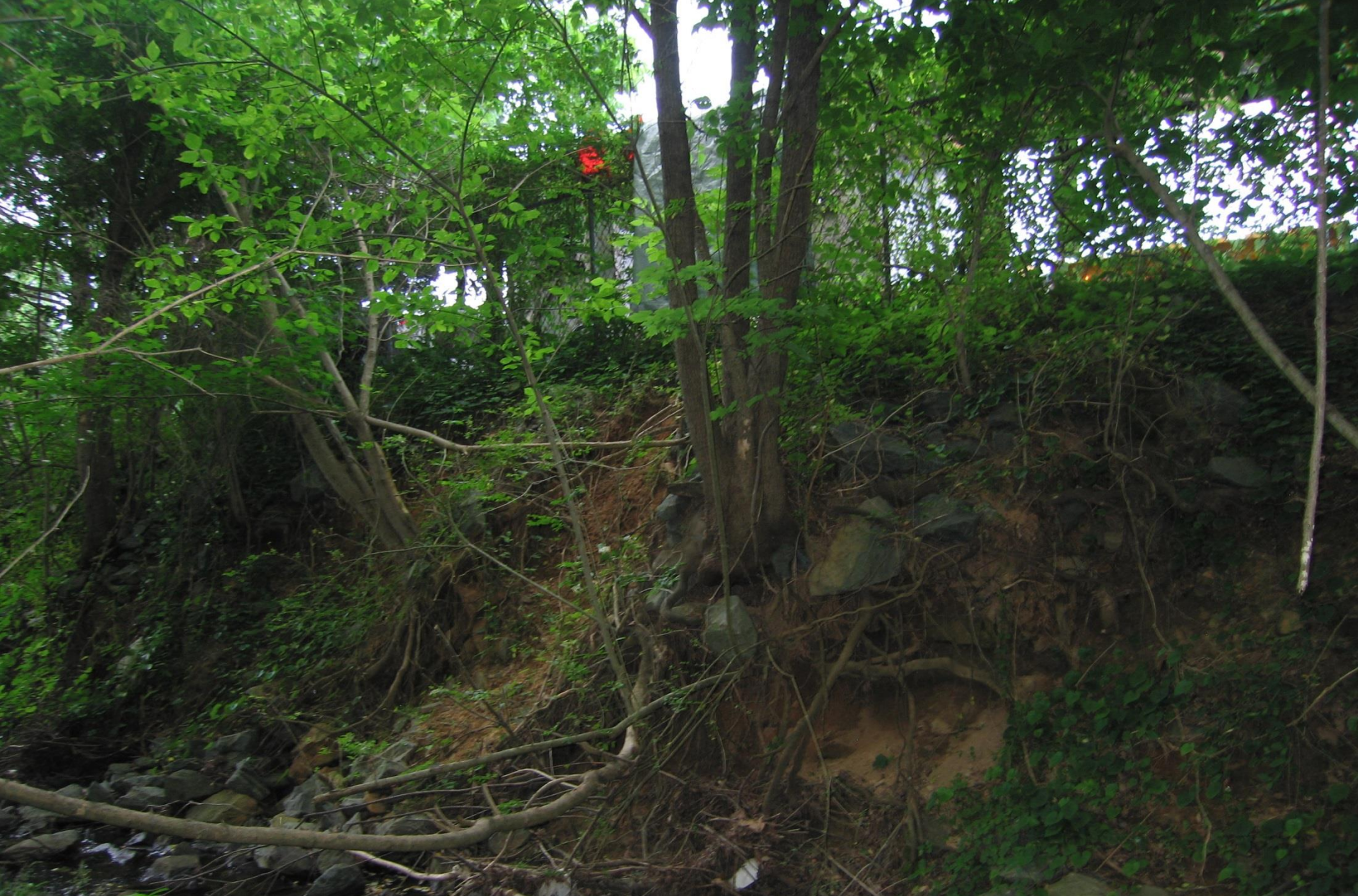
Public Works Drive Inlet – Erosion on Banking near PW Bldgs
