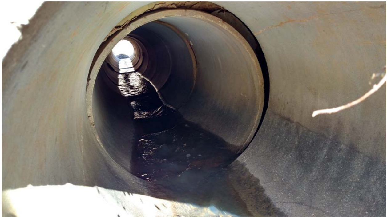
Looking inside 36” Concrete Pipe – Pipe Separation
